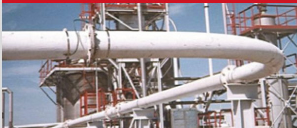
Fig. 10-6 Manufacturing Plant Utilizing Directionally Textured Pipe
